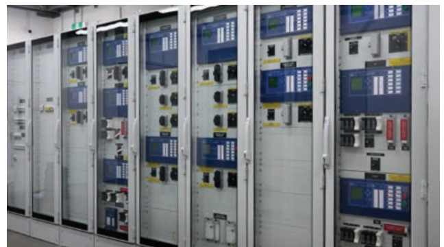
Top image: Ngāwhā 110/33 kV Transmission Substation. Above image: Substation Relay Room.
