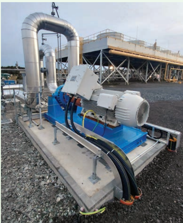
Image: The pump was fully commissioned in February 2026 and is now part of normal plant operations, enhancing resilience and supporting reliable, renewable electricity generation for the Far North now and into the future.
