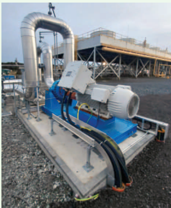
Image: The pump was fully commissioned in February 2026 and is now part of normal plant operations, enhancing resilience and supporting reliable, renewable electricity generation for the Far North now and into the future.
