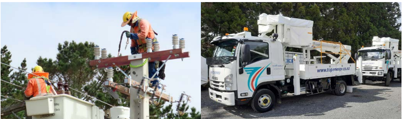
Left: Pole & cross arm replacement at Lake Omapere. Right: Top Energy Elevated Work Platform (EWP) or bucket truck used for everything from vegetation, lines & poles management to cherry picker rides at A&P shows.
