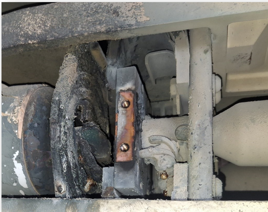
Figure 3: This pair of images shows the L3 phase moving assembly above and the L1 phase moving assembly below note the L3 phase image has been mirrored to provide an equivalent image. Note the severe damage on the L1 phase moving assembly.
