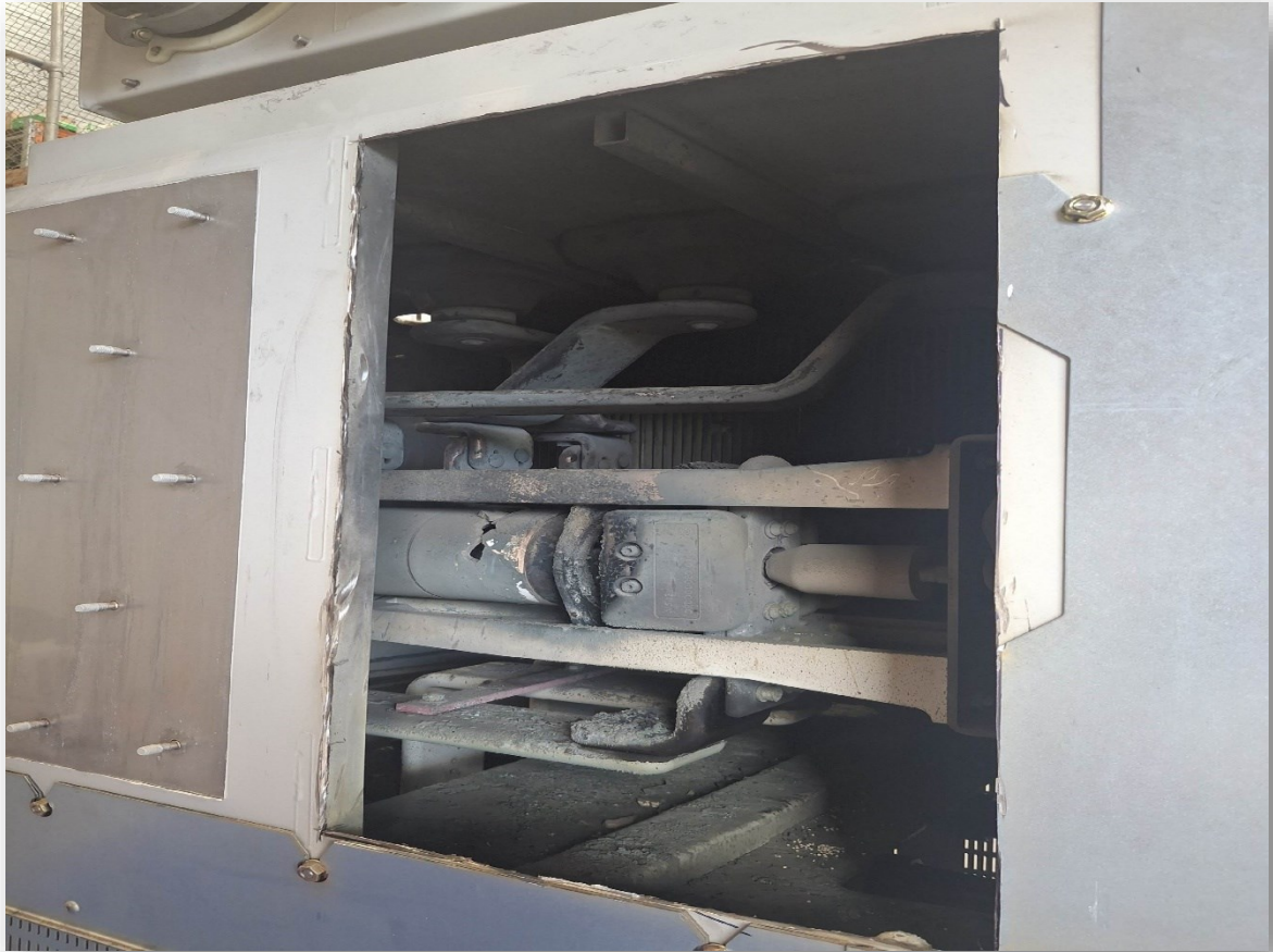
Figure 2: Opening created adjacent to the L1 circuit breaker assembly. Holes in the L1 vacuum interrupter are noted in the middle of the image.
