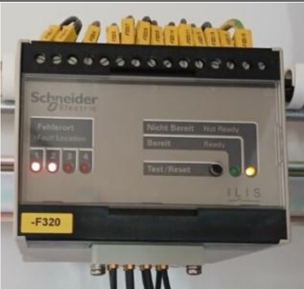
Fig 3: ILIS protection indication for T3 incomer breaker H05 (CB163612)
