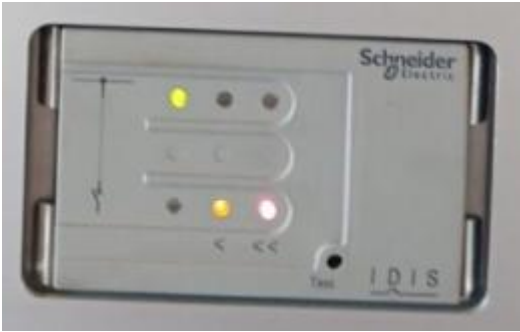
Fig 4: IDIS protection indication for T3 incomer breaker H05 (CB163612)
