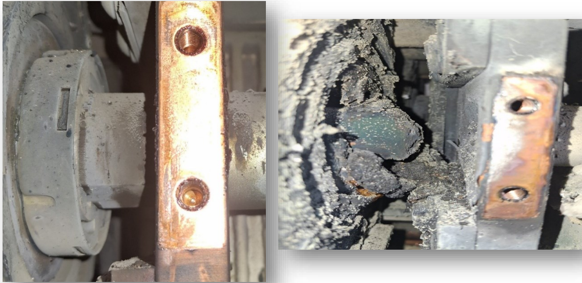
Figure 4: the L1 moving assembly above shows the end of the vacuum interrupter, the stem of the moving contact that is connected to the large copper plate in good condition. The L1 part of the image below shows approximately 20 millimetres of that shaft has been eroded by arcing.
