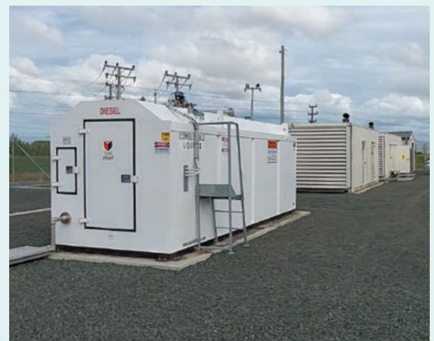
Back-up generators at Kaitaia
