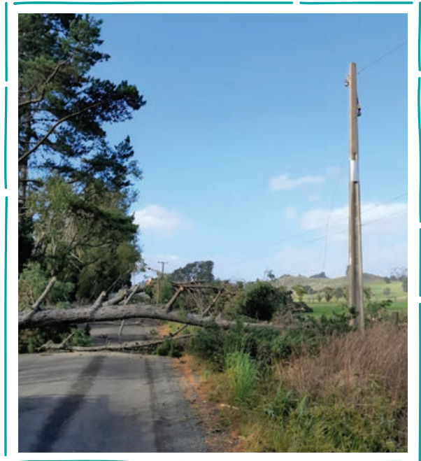
Lines down in Diggers Valley
